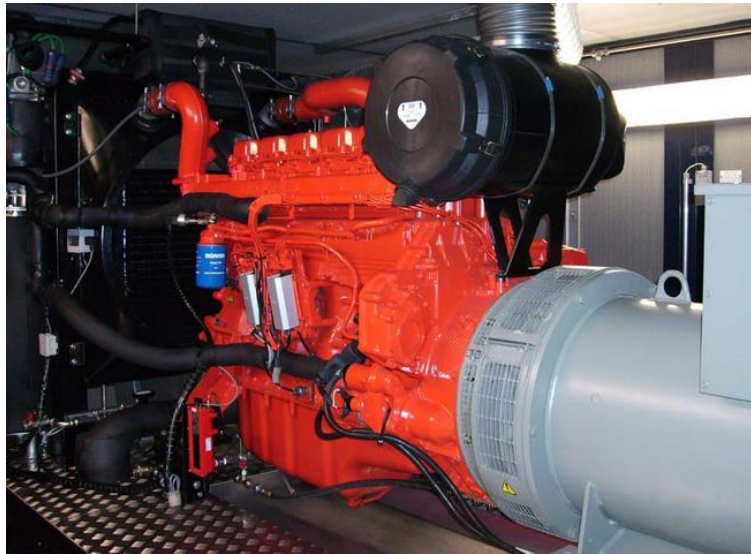
Figure 3.16. The combined heat and power plant supplies the internal energy line
