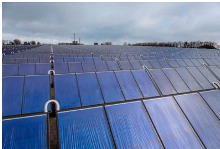
Figure 3.12. Solar energy collectors
