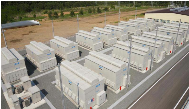
Figure 3.10. Battery storage system (SBC Energy Institute, 2013)
