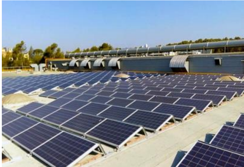
Figure 3.14. Rooftop PV at DENSO manufacturing plant, Barcelona
