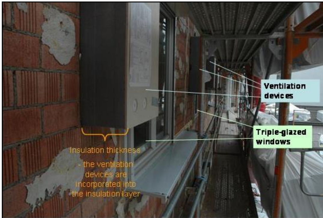
Figure 7.17: Refurbishment of the facade by triple-glazed windows, ventilation devices and 24 cm-insulation layer
